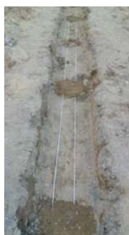
Buried E-Field Sensor
